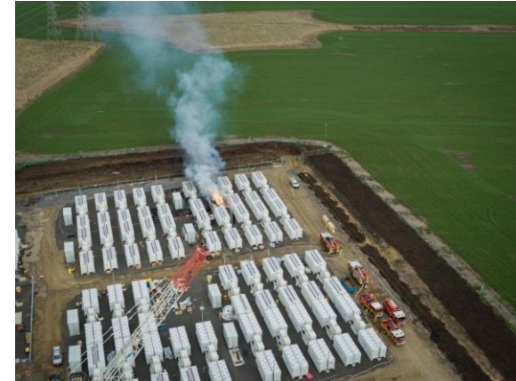
Victorian Big Battery (julio 2021) Australia
